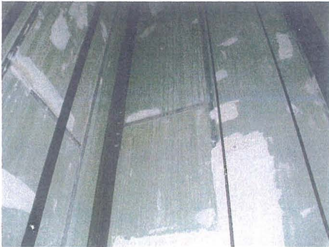
EWR – Newark, New Jersey View of Elevator Shaft Interior
