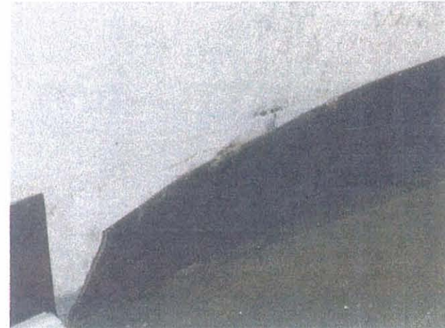
EWR – Newark, New Jersey Suspect Mold Growth Under Cove Base, Ground Floor
