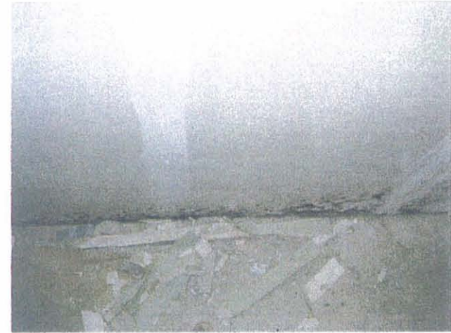
CVG – Cincinnati/North Kentucky Ground Level 8ft 2 Mold Growth in Plenum
