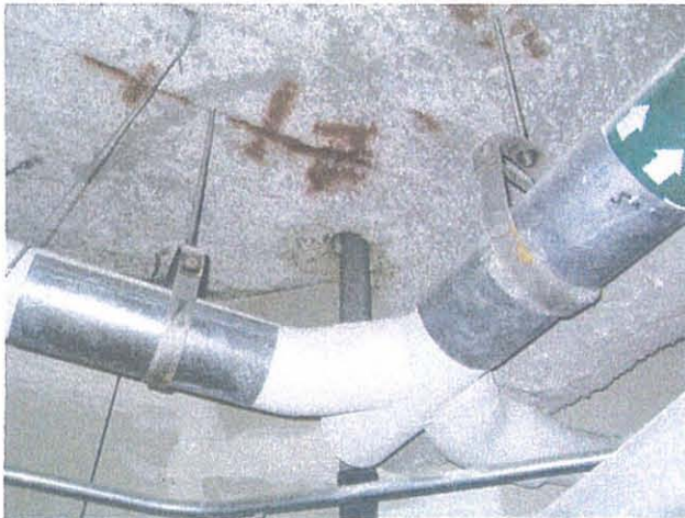
DIA – Denver Subjunction Level Penetration to Microwave Balcony Allows Rainwater to Enter
