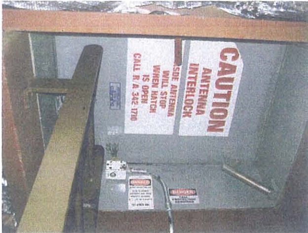
DIA – Denver Penthouse Roof Hatch With Condensation
