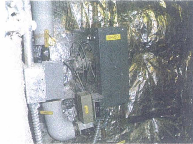
EWR – Newark, New Jersey Convective Heating Unit in Utility Chase
