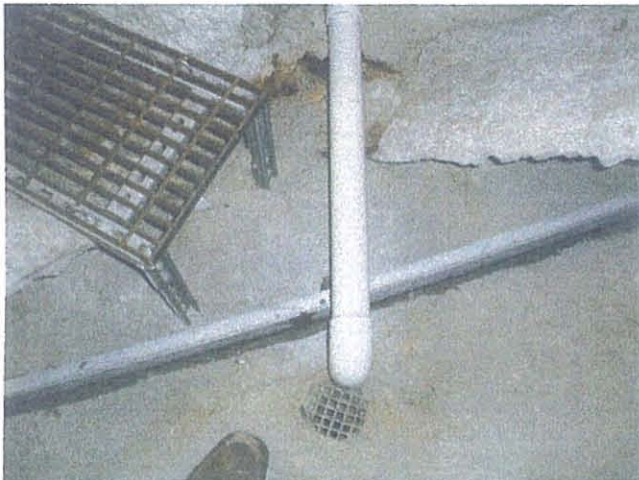
STL – Lambert St. Louis Drain in Air Shaft Modified to Prevent Pooling
