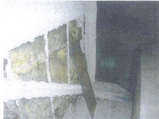
STL – Lambert St. Louis Cable Access Level – Wallboard and Insulation on Inner Ring
