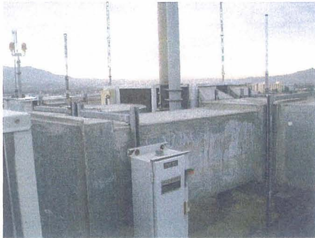
BUR – Bob Hope Burbank Airport Cab Roof HVAC Equipment – Clean and Well Maintained
