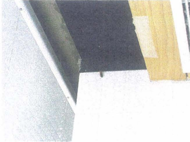
DFW – West Tower Dallas/Fort Worth Junction Level Insect Gains Entrance to Restroom Through Unsealed Crevice
