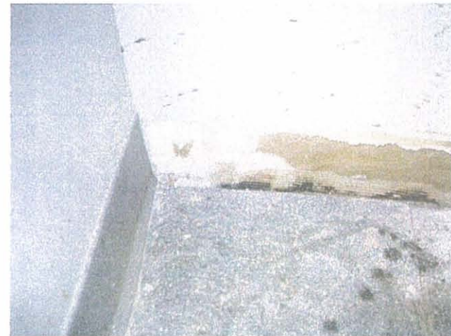
MCI – Kansas City Junction Level Room J10 Small (<6 in 2 ) Patch of Visible Mold Growth
