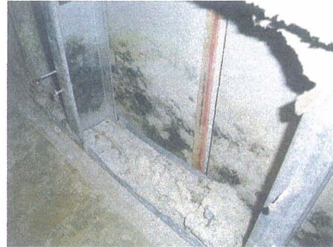
UGN – Chicago Waukegan Regional Visible Mold Growth Inside of Wall – First Floor Elevator Lobby
