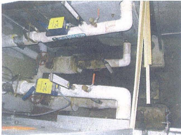
ORD – Chicago Mechanical Room Leaking Valve Repaired During Survey
