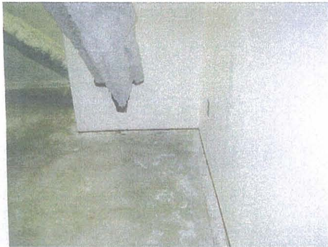
MCI – Kansas City Typical Mold Abated Wall Area
