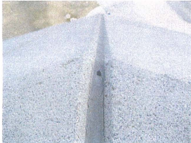
AUS– Austin Cab Balcony Deteriorated Seam Caulk
