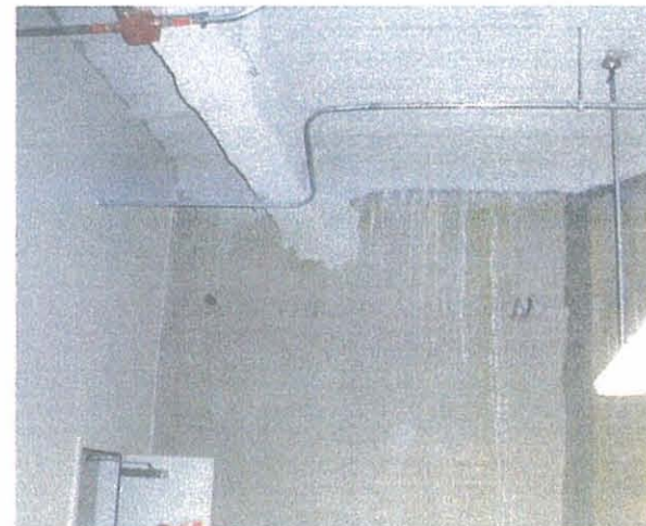
SEA – Seattle Tacoma 10 th Level Typical Wall Staining Likely From Original Fireproofing Application
