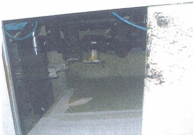
IAH – Houston 11 th Level Fitness Room Condensation on Chilled Water Valve and Affected Ceiling Tile
