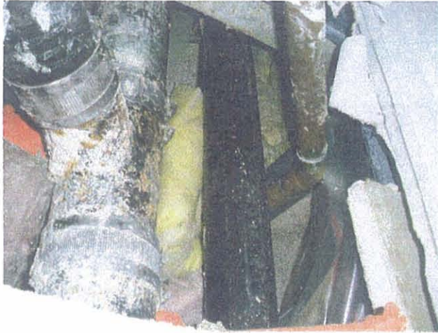
UGN – Chicago Waukegan Regional Opened Vertical Pipe Chase With Inadequate Thermal Insulation
