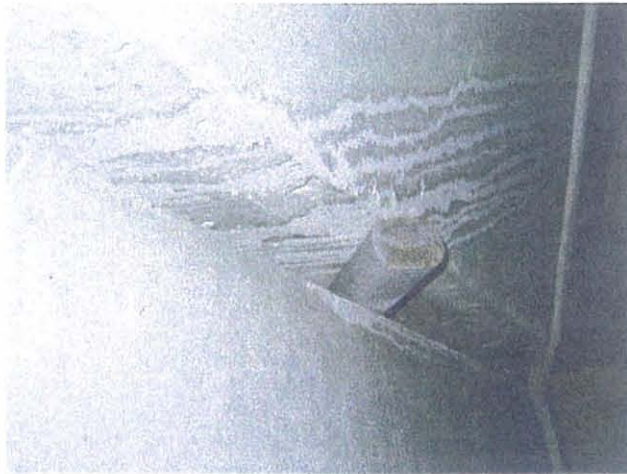
CVG – Cincinnati/North Kentucky Cable Access Level Exterior Wall With Water Stains
