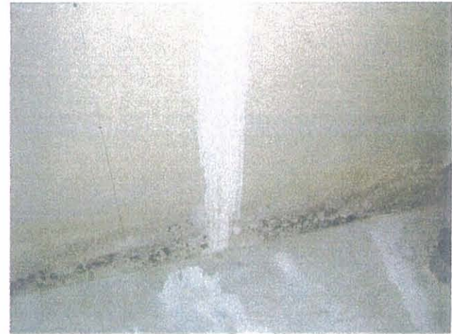
DFW – East Tower Dallas/Fort Worth Non-functional Area Mold Growth
