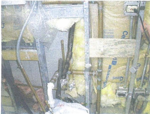
UGN – Chicago Waukegan Regional 5 th Level Domestic Water Line Burst Creating Flooding of Tower
