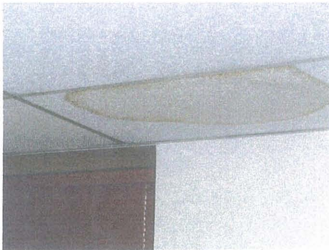
BUR - Bob Hope Burbank Airport 6 th Level Ceiling Tile Stain From Sanitary Drain Line
