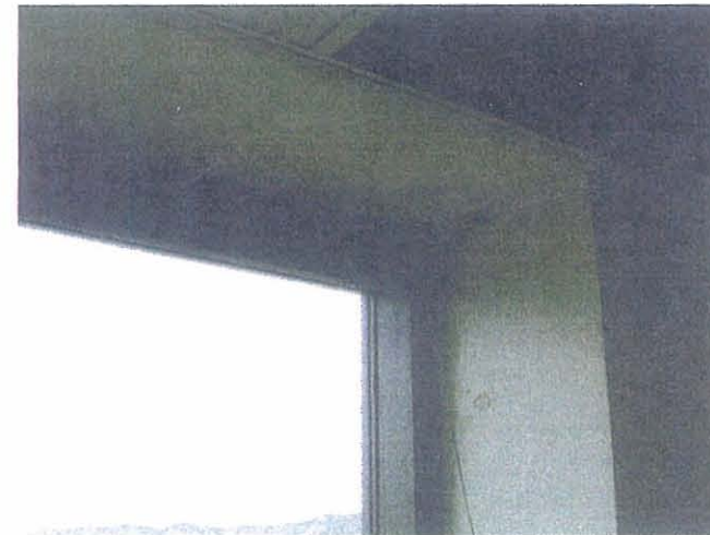
BUR - Bob Hope Burbank Airport 3 rd Level – Small Amount of Mold Growth Near Window Which Was Re-caulked
