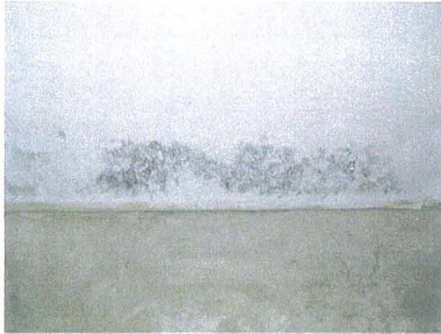
IAH – Houston Room 2S3 Mold Below HVAC Duct
