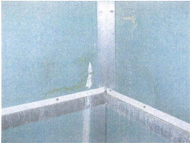
DFW – East Tower Dallas/Fort Worth Elevator Shaft Mold Spotting and Water Stain
