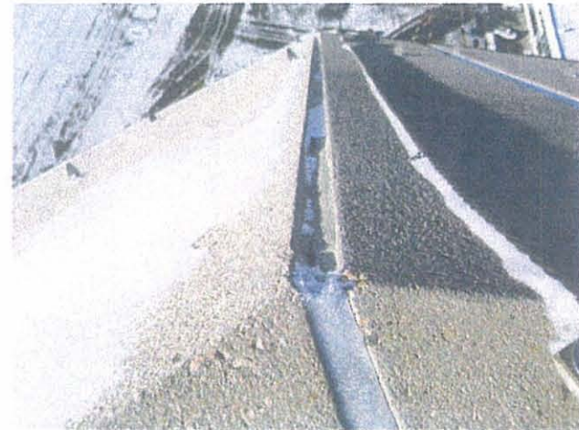
DIA – Denver Cab Balcony Deteriorated Seam Caulk
