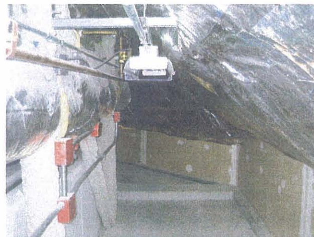
SDF – Louisville Cable Access Level Insulated Exterior Wall and Metal Structural Members
