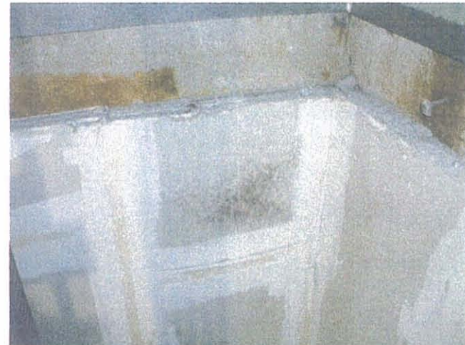
STL – Lambert St. Louis Suspect Mold Growth in Elevator Shaft
