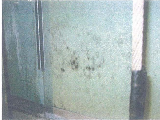
AUS – Austin Mold on Green Board Paper in Elevator Shaft
