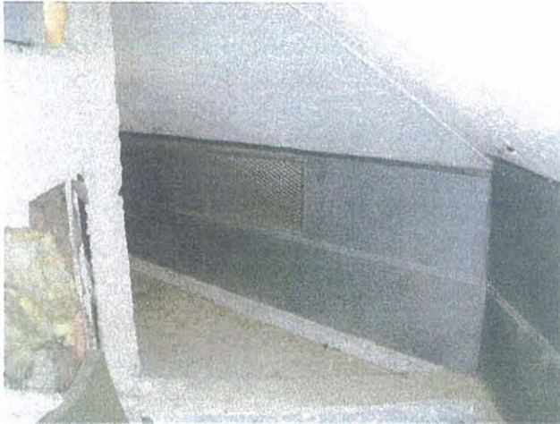
STL – Lambert St. Louis Cable Access Level – Uninsulated Perimeter Walls with Vents to Outdoors
