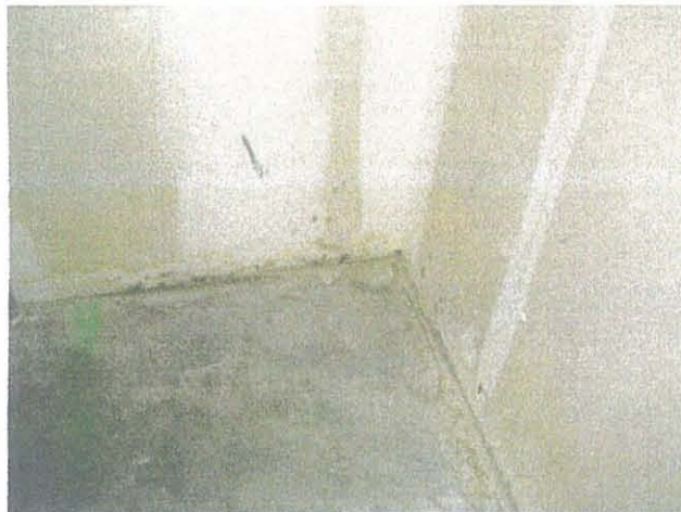
CVG – Cincinnati/North Kentucky Room 8TS3 Mold Growth and Water Stained Wall
