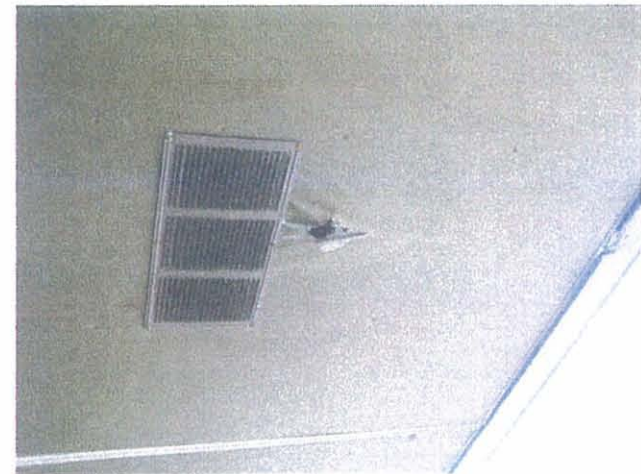
CVG – Cincinnati/North Kentucky Junction Level Balcony Water Damaged Soffit
